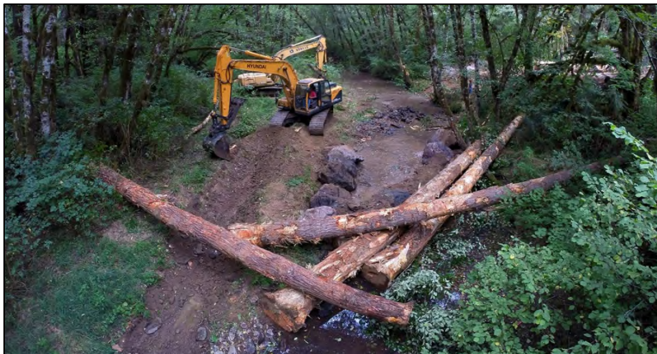
Figure 5.15. Large equipment use on a forest stream restoration project. Source Oregon BLM.
